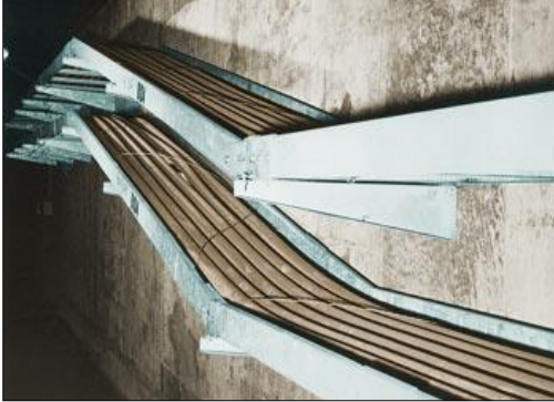
Sensor cable installed inside a cable tray
