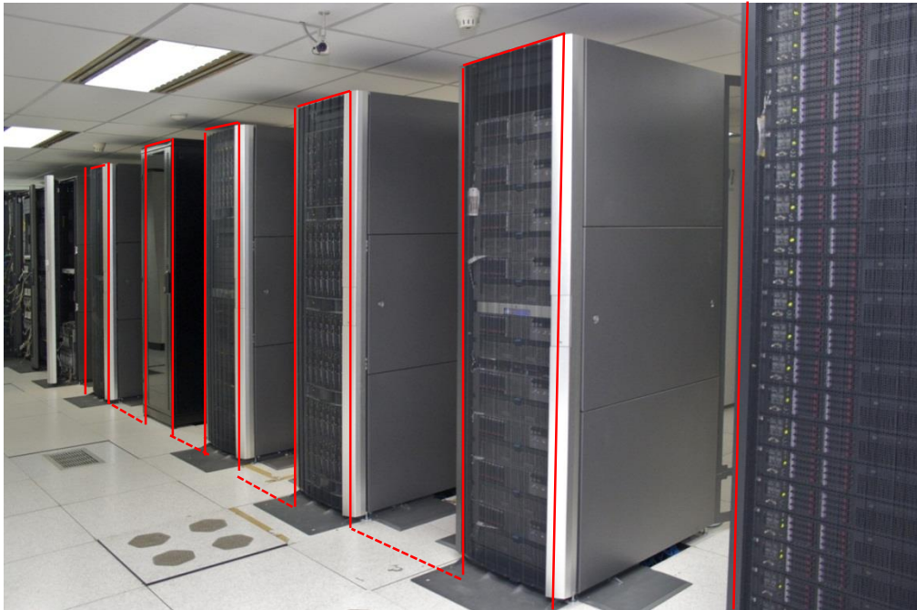
Passive sensor cable detects hot and cold spots on the racks, in the aisles and below the floor
